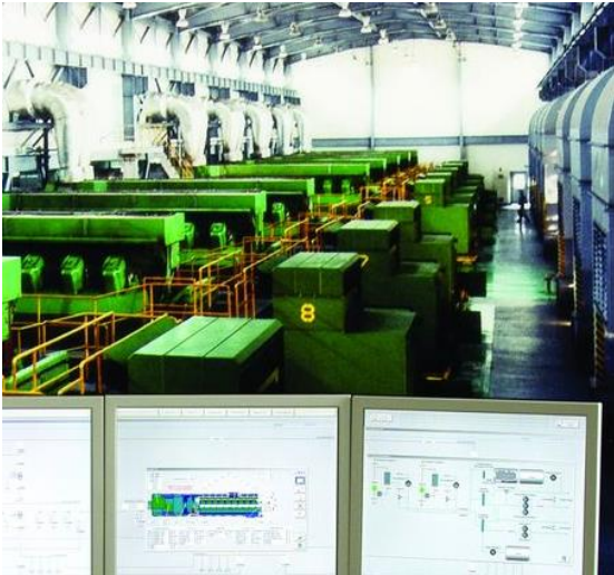
Diesel/Gas Engine Power Plant
