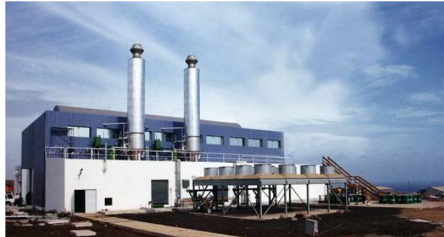
Gas/Steam Turbine Power Plant
