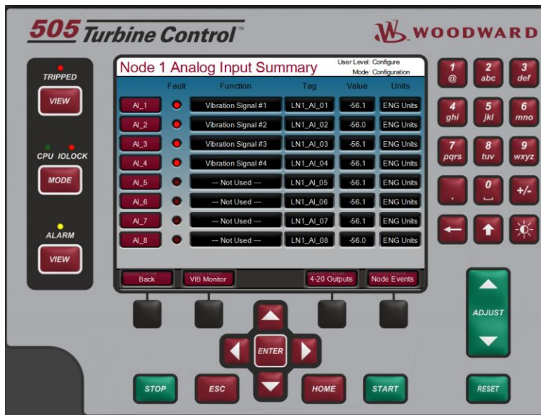
Figure 1-8. LinkNet Node 1 with 4 Vibration Signals
