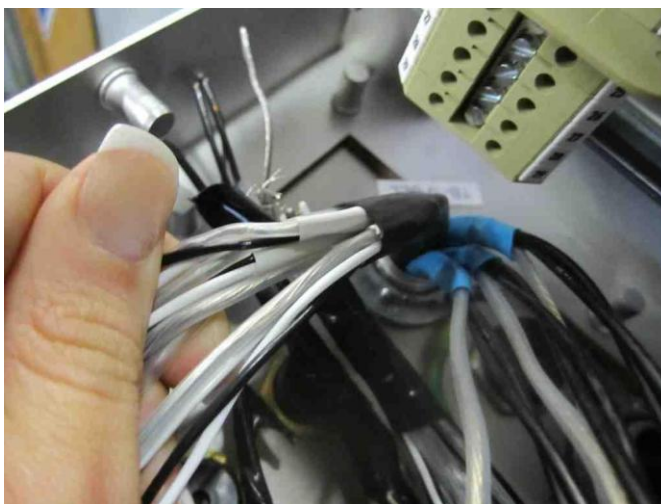
Figure 3-5. GS40 Analog/Drain Wiring Prep
