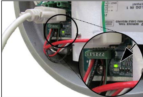
Figure 6-3. CPC-DX with applied electrical power – green LED illuminate.
